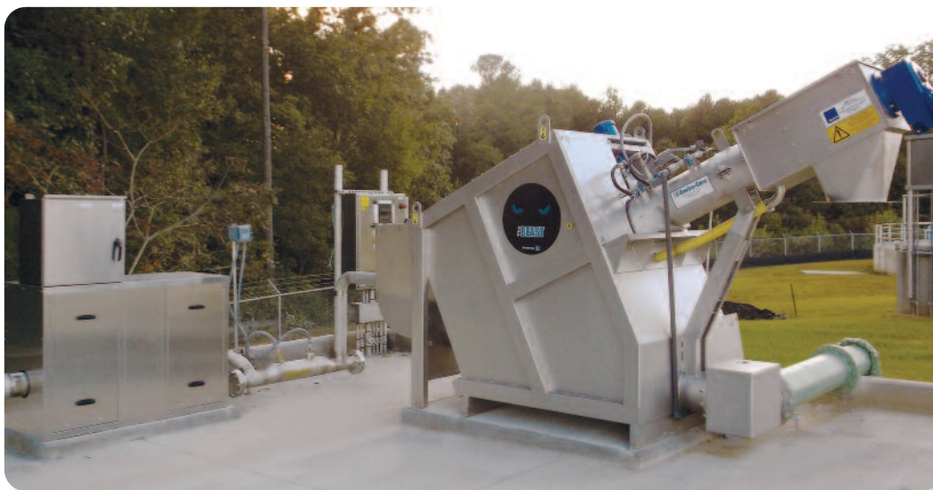
Kershaw County South Carolina BEAST Septage Receiving Station
