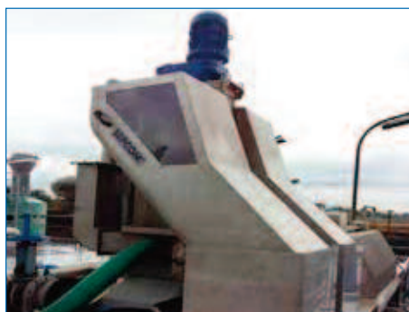
Waste water treatment plant (SEPCOM Industrial Vertical)
