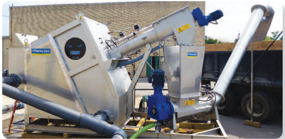
Screened sludge being dewatered by an SAVI® VWP-3 Washer Compactor.
