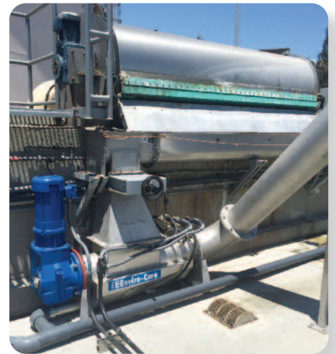
A SAVI® VWP-2 Washer Compactor receiving screenings from a launder system.
