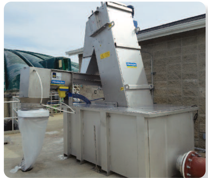
Fish Creek WI In Tank Unit Feeding a SPECO® Conveying Compactor.
