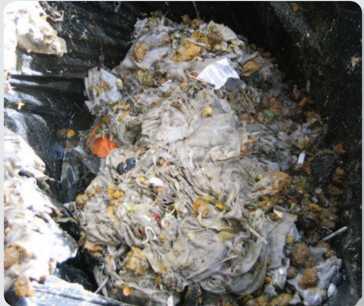
Screenings Removed by the Flo-MultiRake Fine Bar Screen
