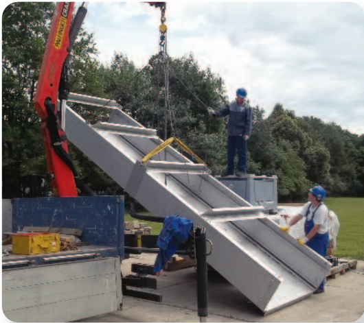
Field assembly of long MultiRake Screen.
