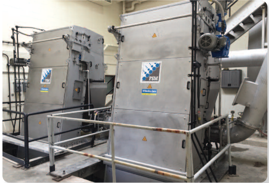
Rock River Water Reclamation District
