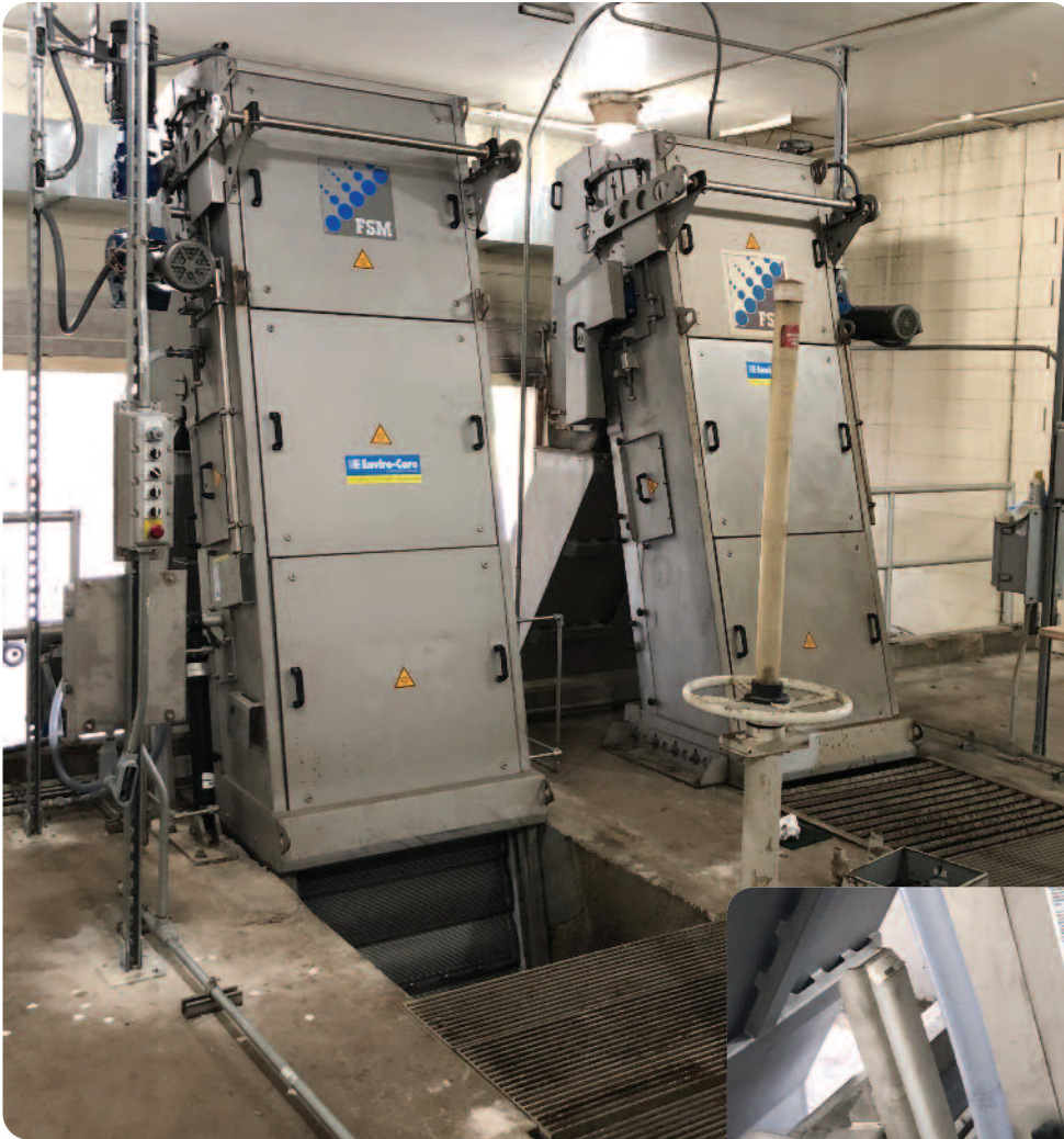
Beaver Dam, WI - Lifting System
